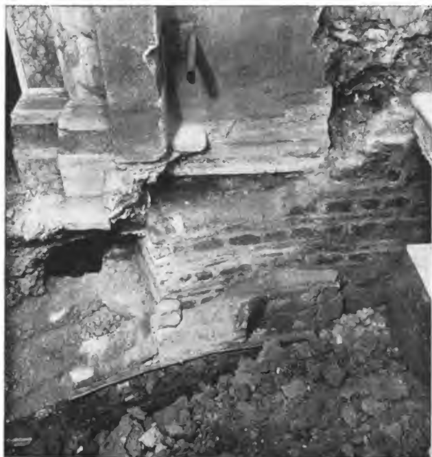
Fig. 42 — S. Lorenzo f.l.m. Excavations 1947-49. Apse H, northeast springing from south, and window jamb (Photo: Sansaini).
